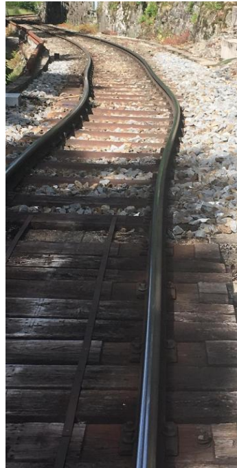
Railway track deformation
